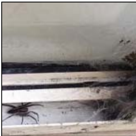
Debris in the window track
