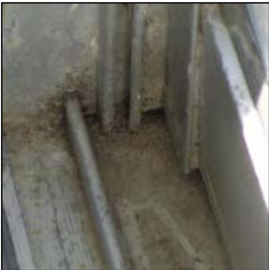
Failing corner joint
