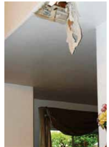
Loose drywall tape and plaster is typically not a serious health risk.
