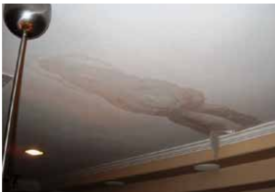
Standard ceiling leak
