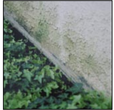
Stucco buried by planter
